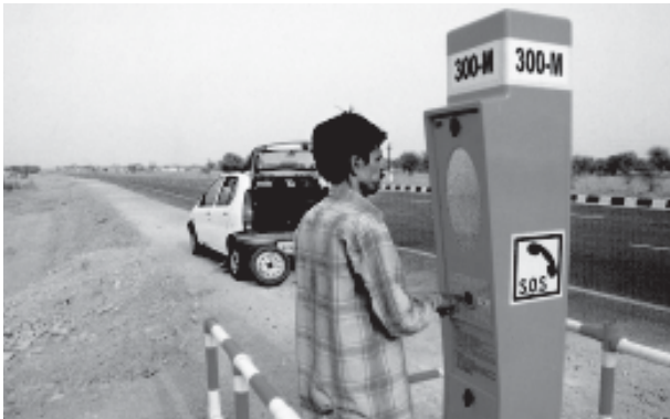
Fig.7.10 : Emergency call box on NH-8
