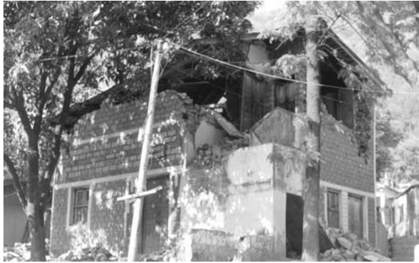
Figure 7.1 : A Damaged Building Due to an Earthquake
